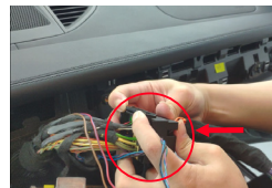
11. Take out the CarPlay main line and connect the CarPlay main line with original car main line
